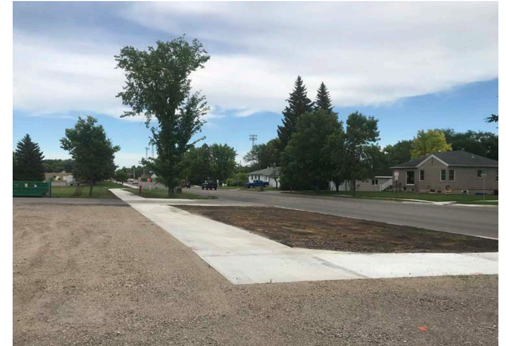
A shared use path that was recently constructed along the north side of 15th Avenue North, which connects to the southern terminus of Gap 16.
